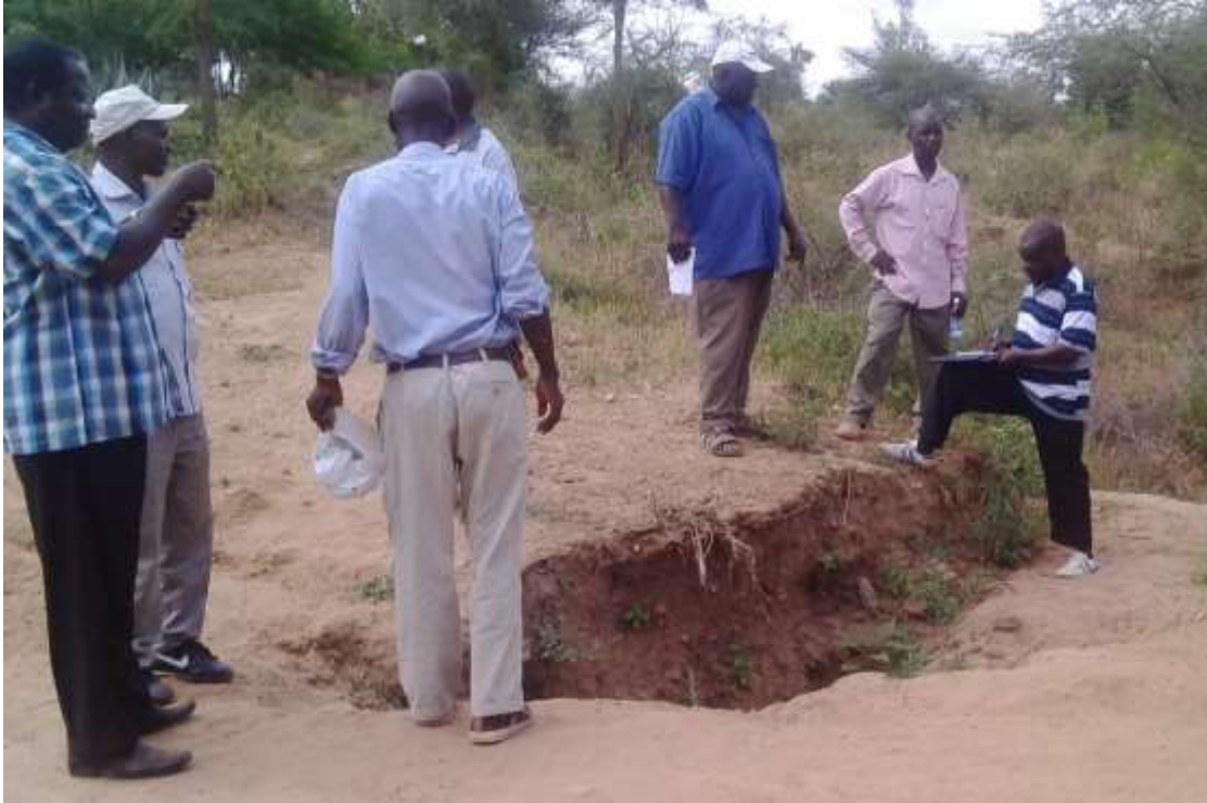
Figure 11 A poorly installed culvert along Kitui – Kwa Masesi-Imale Road.
