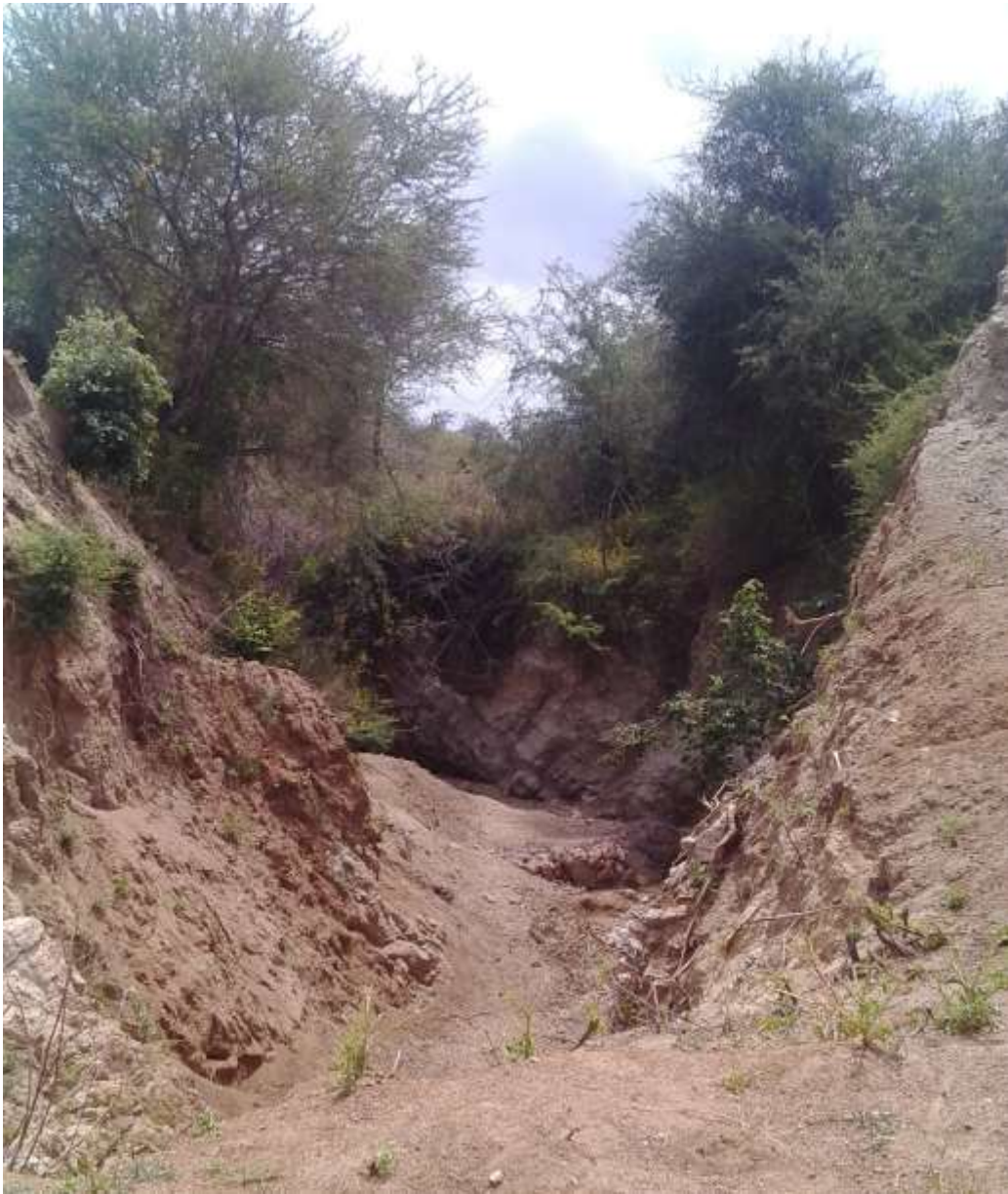
Figure 4 Poorly designed Kwa Mukai earth dam.
