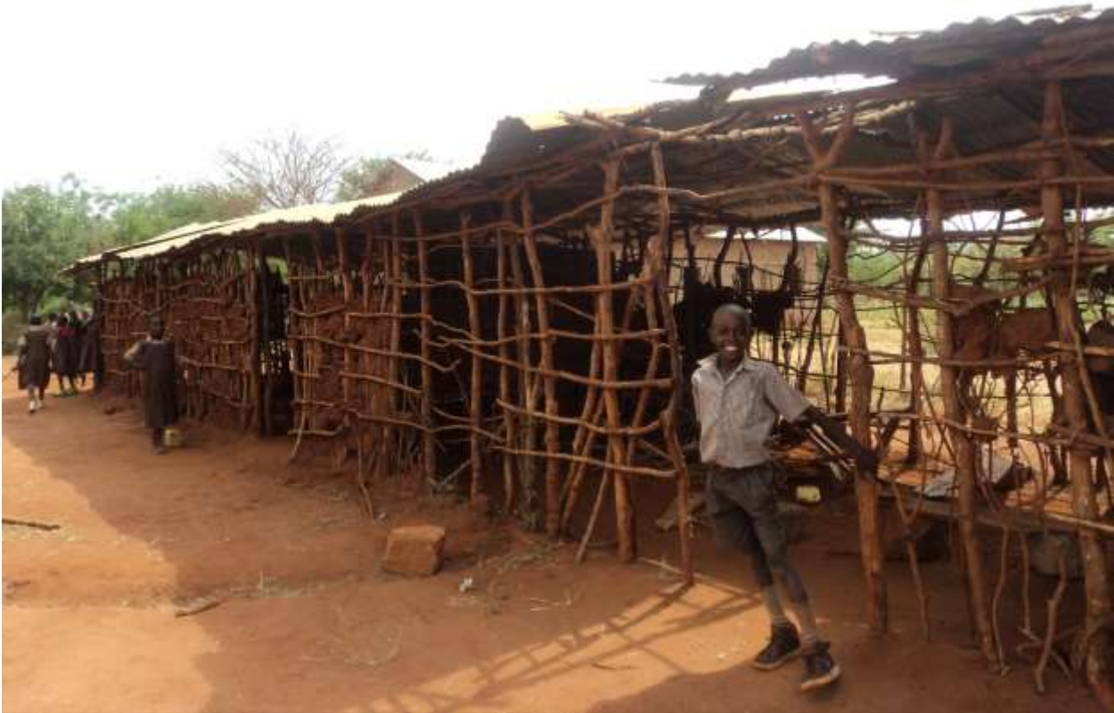
Fig. 7 Section of the dilapidated classrooms at Maweli Primary School.
