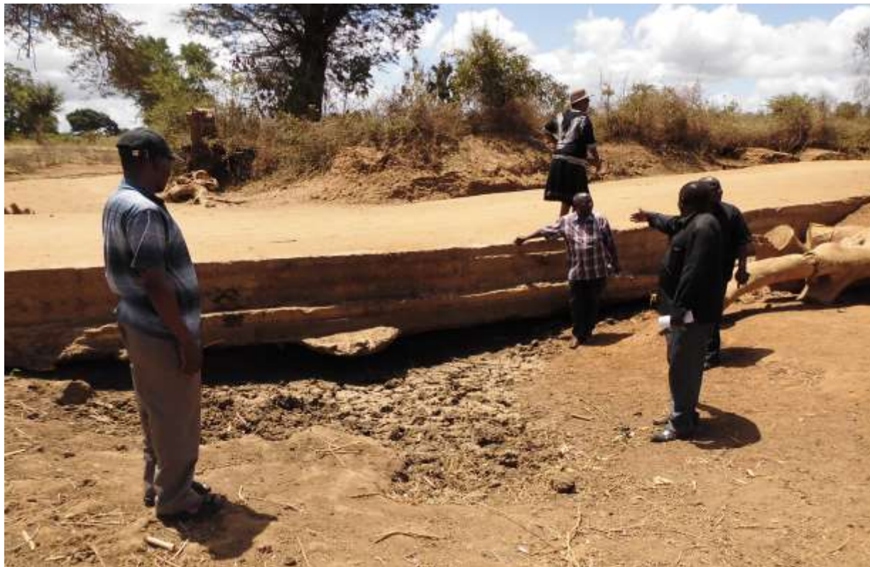
Photograph 2: A suspended drift poorly done on Kitungati - Kamulu Road in Mbitini Ward
