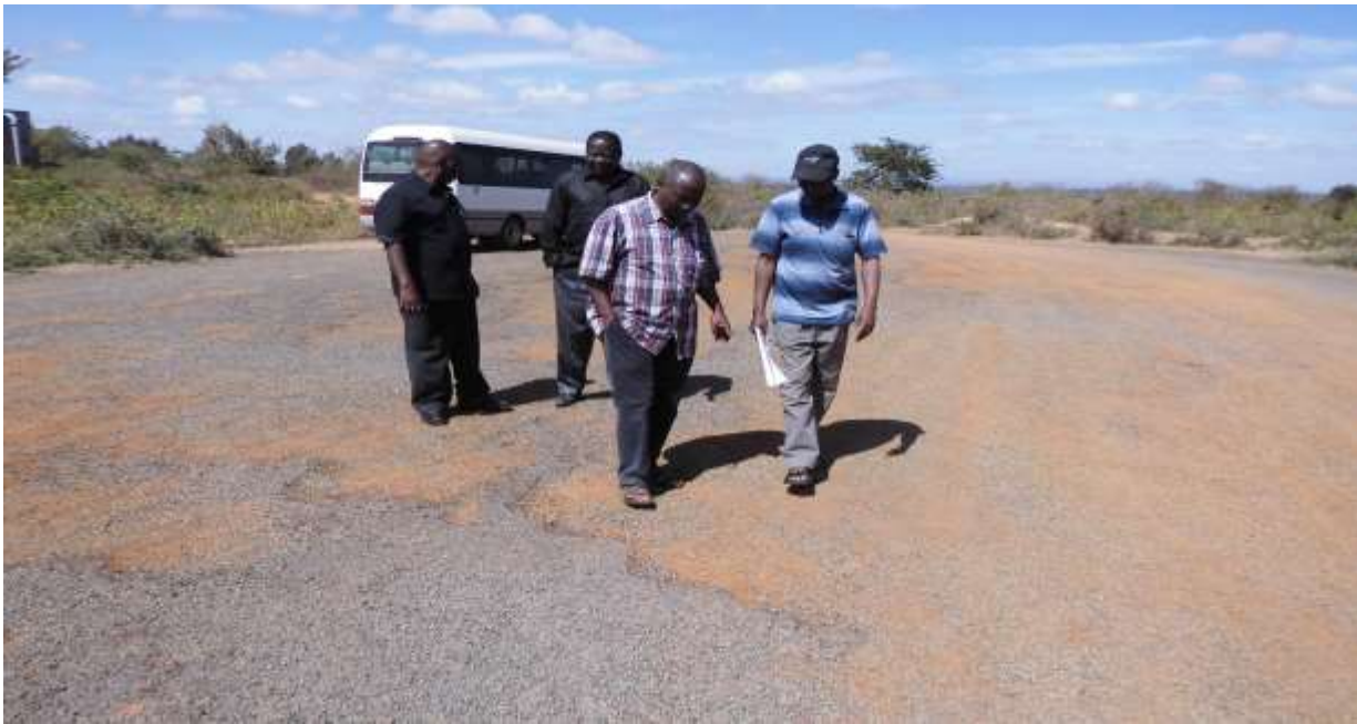
Photograph 1: Assessment of the badly dilapidated Kitui Airstrip at Ithookwe, Kyangwithya West Ward
